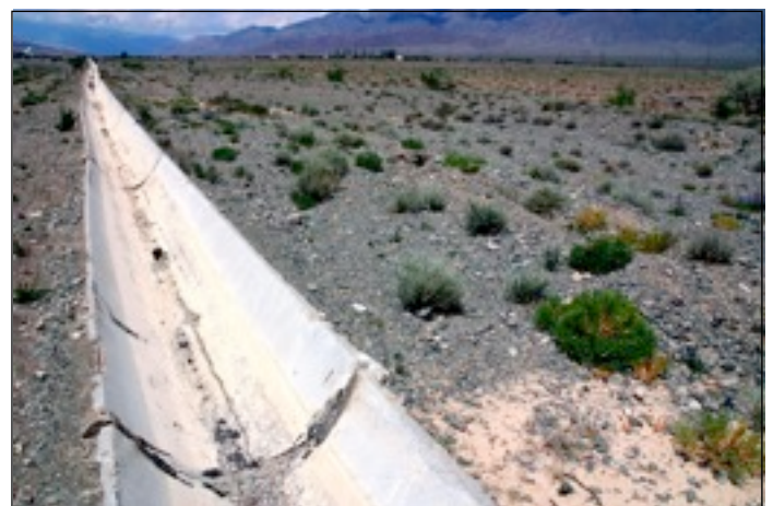
7.103 This Soviet-era irrigation canal near Lake Issuk-Kul in Kyrgyzstan has fallen into disrepair. Large sections of the concrete structure have been stolen by local people for use as building materials.
