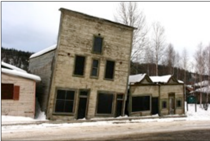
7.148 These buildings in Dawson City (Yukon, Canada) show what can happen when heated buildings are placed on frozen permafrost ground. The permafrost melts, mixing soil with water forming a paste into which the footings settle at different rates.
